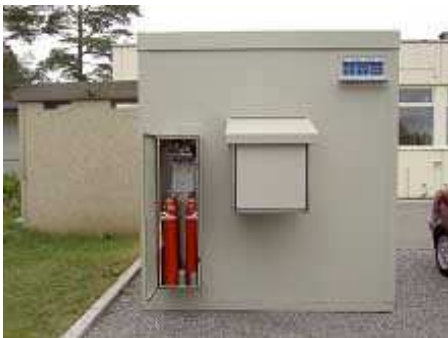
Example of an outdoor hydrogen installation
